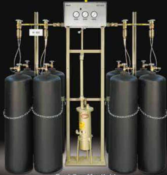
Fuel Gas Manifold
