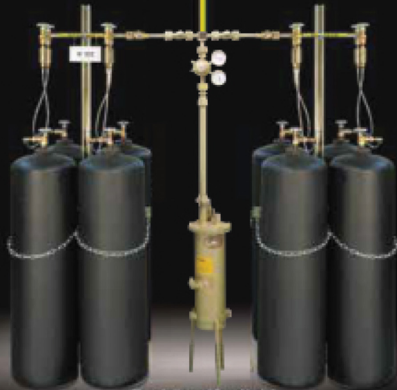
Fuel Gas Manifold
